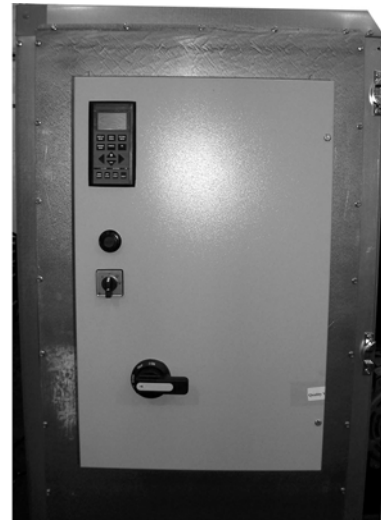
Figure 59. Variable-frequency drive (VFD)
